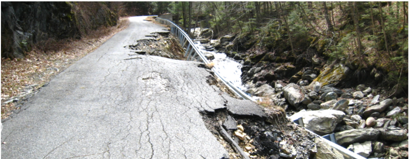
Figure 9: Hurricane Irene severely damaged Black Brook Road in the fall 2011.
